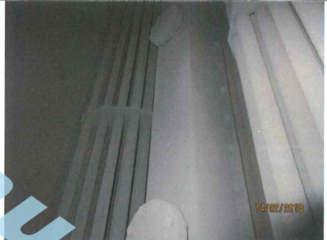
Inside economizer (S-side)
