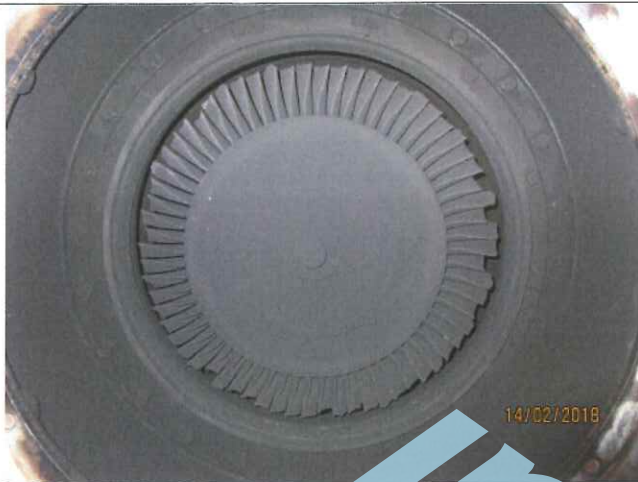
T/C turbine blades (damaged)
