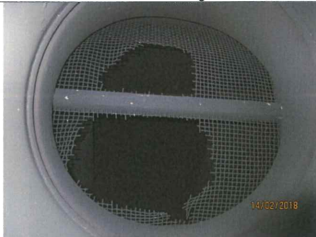
T/C gas inlet, mesh broken.
