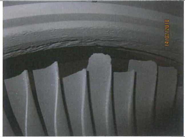
T/C Turbine blades damaged (Details)
