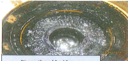
Dismantling of Fuel Pumps Found Oil Sludge on Barrel top side
